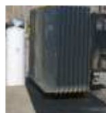
Ideal underneath leaking transformers.
