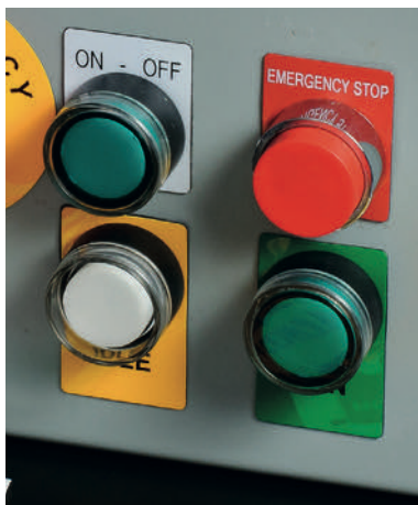
Control panel labels
